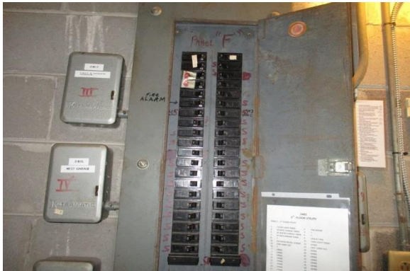
21 Breaker Panel Overview
