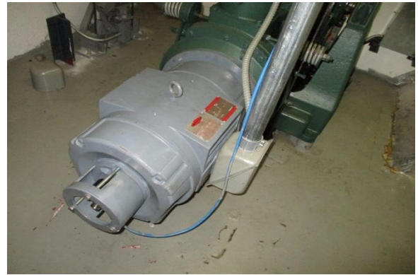
18 Elevator Motor Overview
