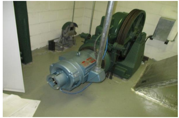
26 Elevator Motor Overview
