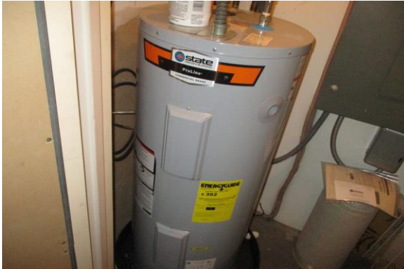
27 Water Heater Overview
