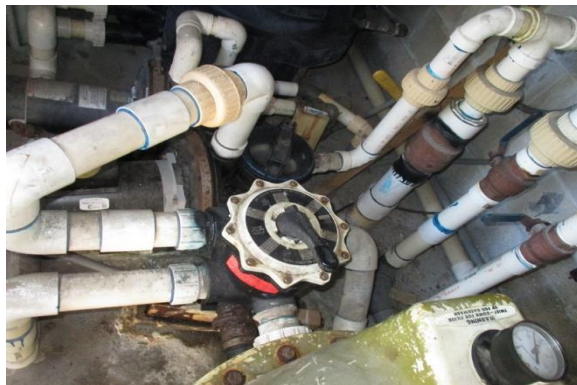
31 Pool Pump Overview
