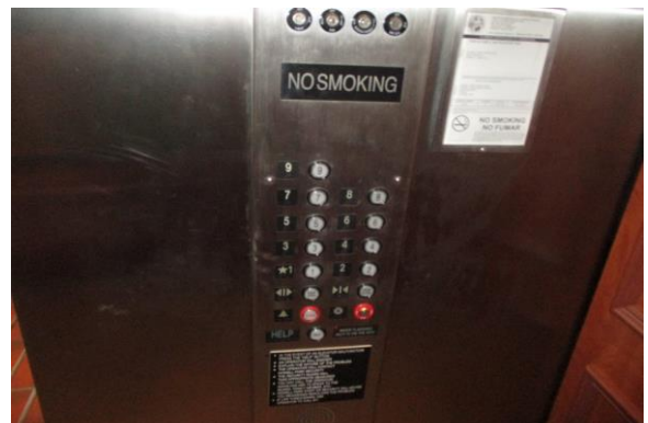
16 Elevator Control Panel
