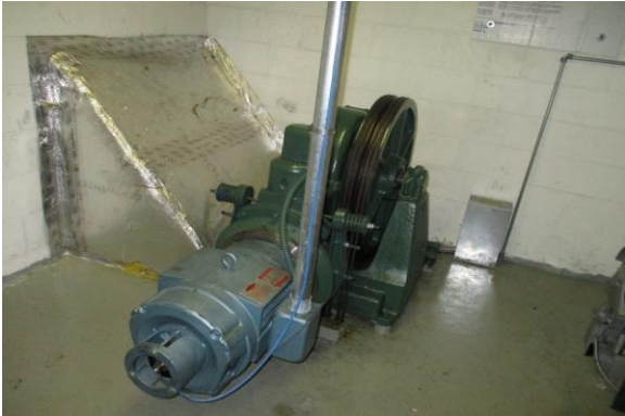
19 Elevator Motor Overview
