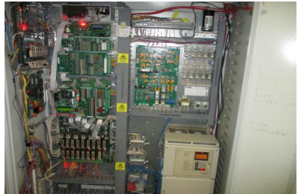
20 Elevator Circuit Board
