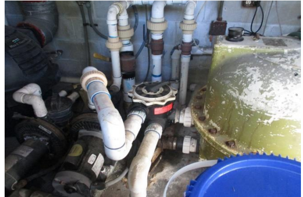
30 Pool Pump Overview
