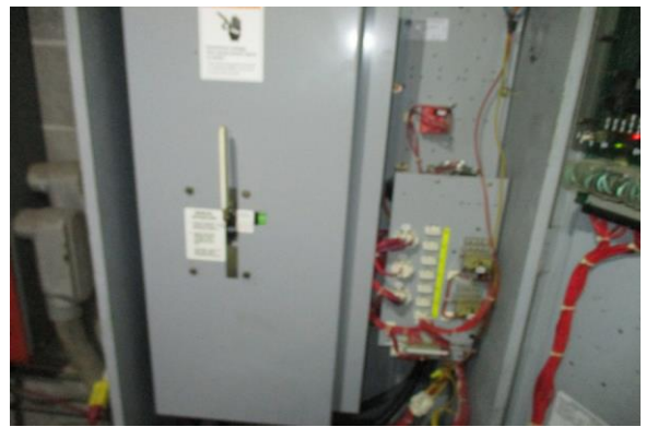
18 Transfer Panel Overview
