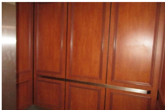
15 Elevator car Overview
