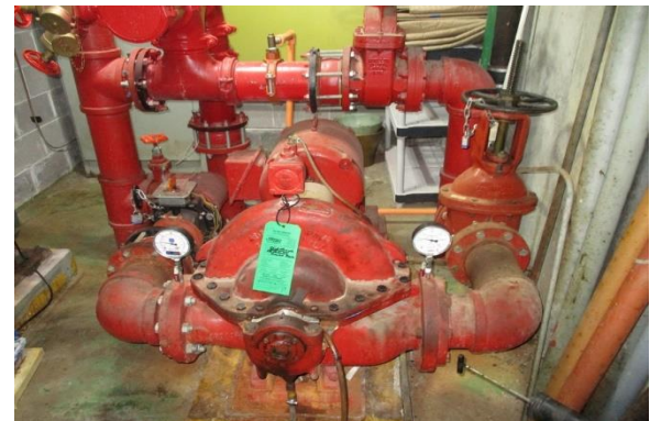
22 Fire Pump Overview
